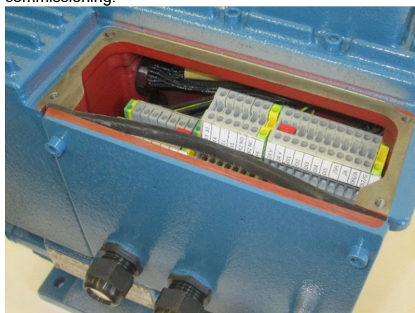
Compact driver terminal compartment
